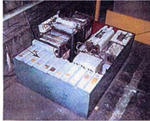
Stored PCB-containing stabilizers
