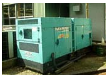
Captive power generation for air conditioning
