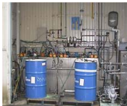
Recovery and recycling equipment for mold releasing agent
