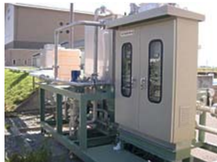
Sludge reduction system
