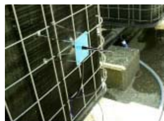
Improvement of heat exchanger efficiency
