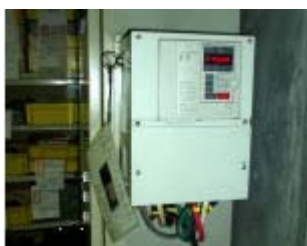
Inverter-controlled water pump
