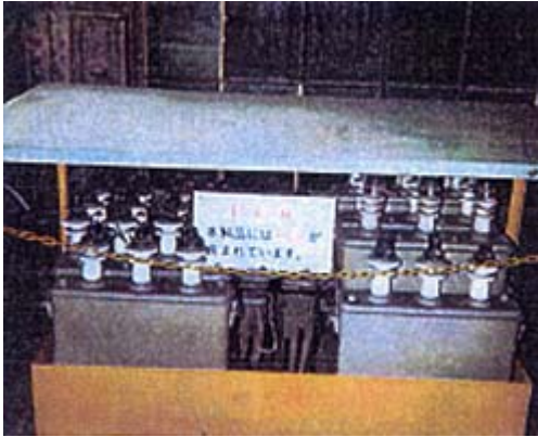
Stored PCB-containing condensers
