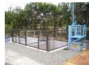
▲ Rainwater Discharge Outlet Oil/Water Separator Tank
