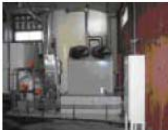
▲ Chilled Seawater Making Equipment
