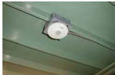
▲ Installation of Infrared Light Timer Sensor
