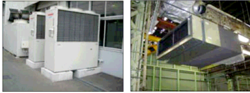
▲ Outdoor GHP units 20PS x 2 units ▲ Indoor GHP unit
