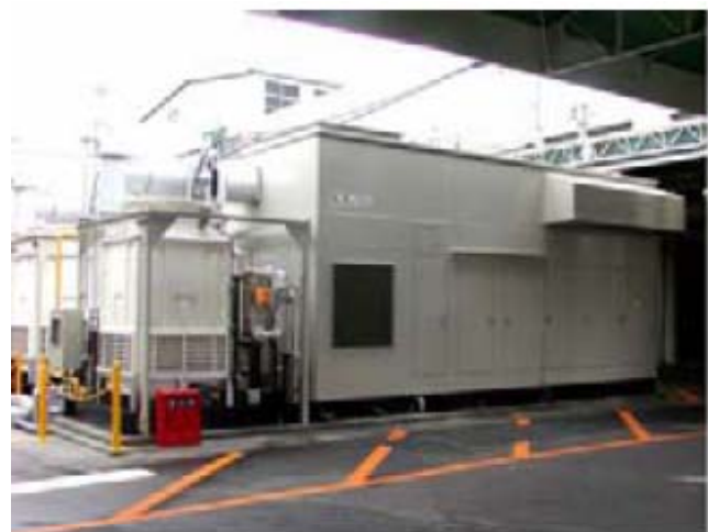
▲ Overall view of gas cogeneration facility
