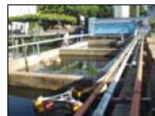
▲ Water Discharge System Oil/Water Separator Tank
