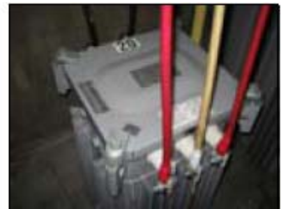
▲ Single phase, 20KVA
