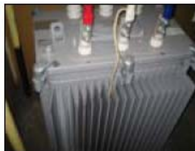
▲ Introduction of high efficiency transformer, 3-phase 100KVA
