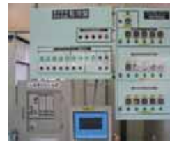
Compressor Control Unit
