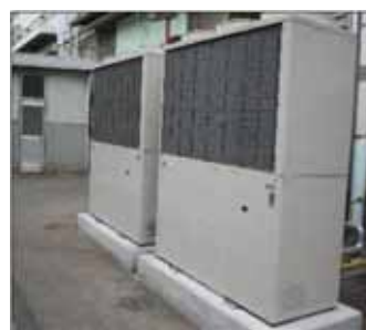
GHP Outdoor Unit in the 7 th Plant, 20PS x 3 units (One unit not shown here)
