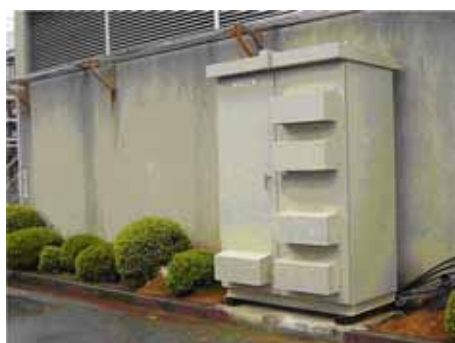
Low voltage electric box
