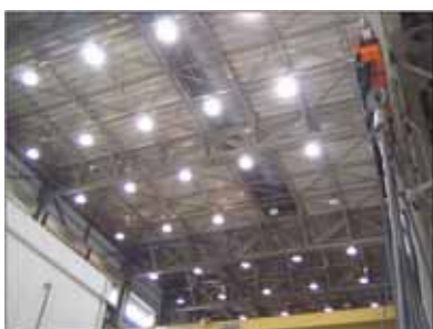
Energy saving mercury lamps in the 8 th Plant, 60 units
